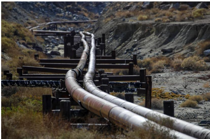
Water pipes, owned by Searles Valley Minerals, snake through Poison Canyon along Highway 178 in Trona. (Irfan Khan / Los Angeles Times)
