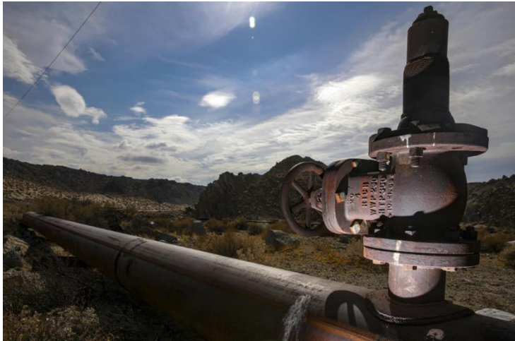
A pipe owned by Searles Valley Minerals carries water to a plant where it is used in the production of soda ash, boron and salt.
